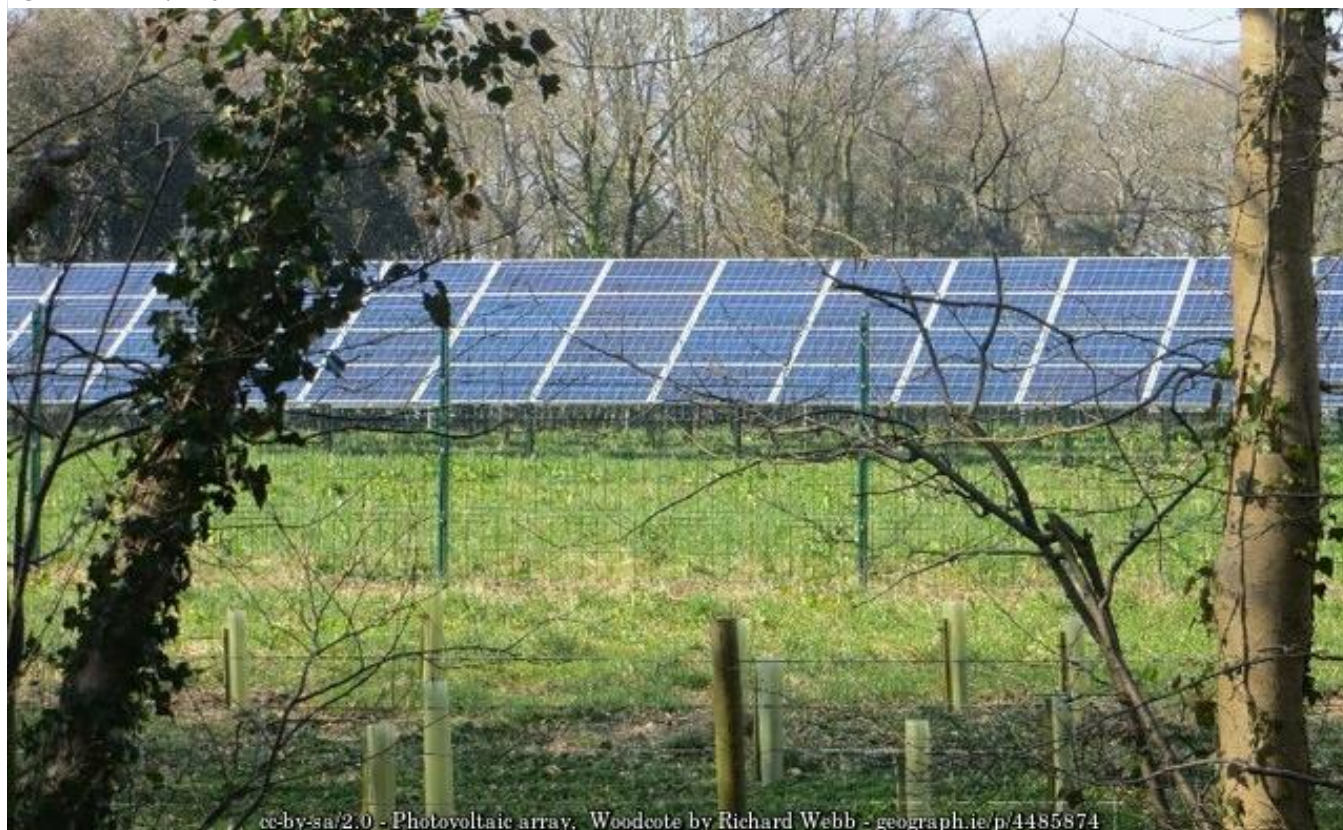
Figure 15: Example of Solar Farm in Woodcote, Devon
