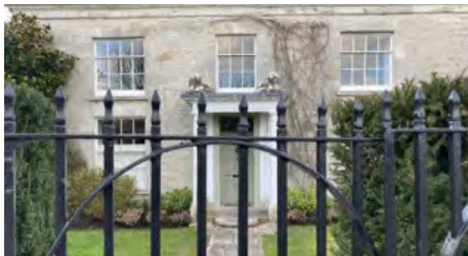
Figure 13: Portesham House with boundary wall made of stone rubble with refined chamfered tops
