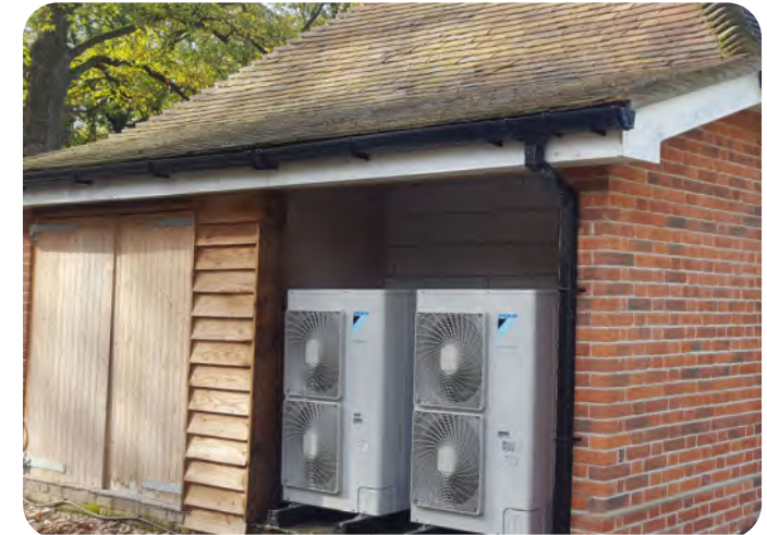
Figure 63: Place pumps in a recessed space to minimise the visual impact
