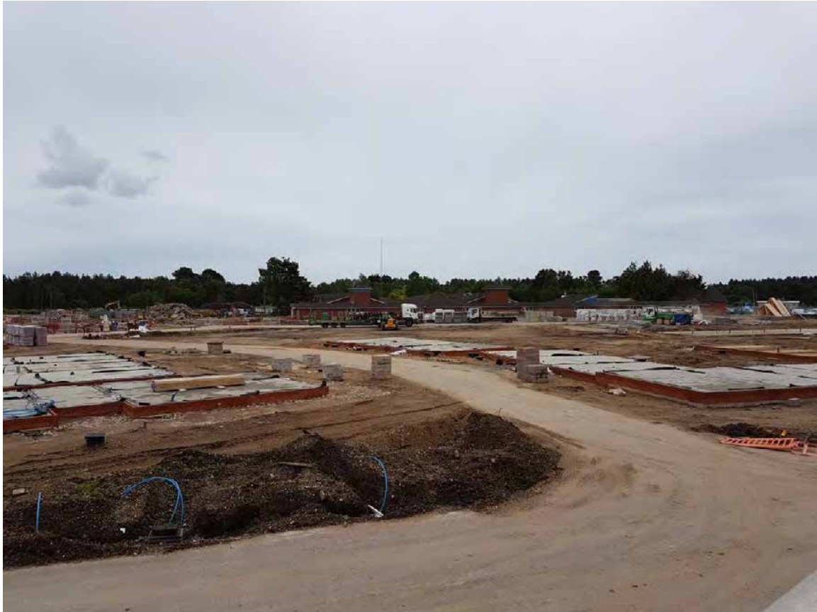
The Victory Oak development under construction, viewed from the A31 footbridge, with Hurn Forest behind
