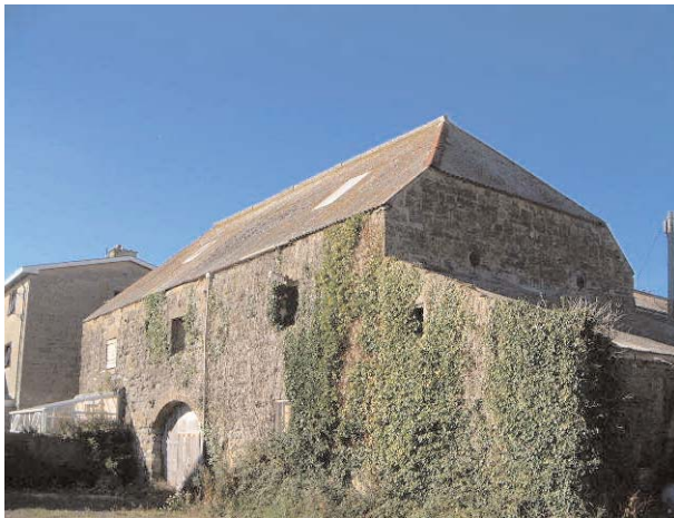
The building on the corner of George Street and West Bay road
