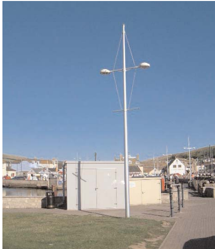
An example of the new harbour and esplanade lighting columns
