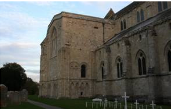
Figure 7: The Priory Church which may incorporate the remains of the late Saxon Minster.
