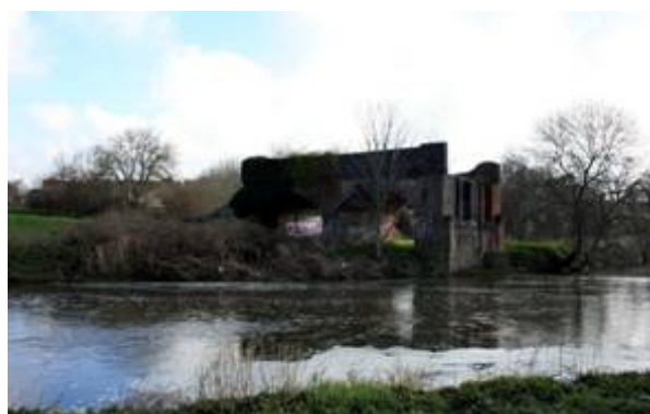
Figure 40: A short surviving section of the former railway bridge over the River Stour.
