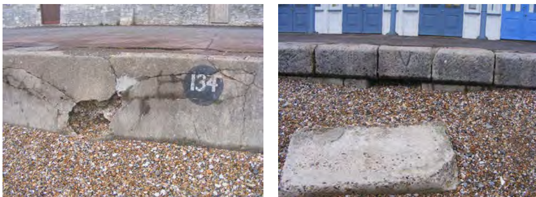
Figure 3-17 Evidence of voids behind damage in the seaward face of the seawall (23-11-2018; photos by A. Frampton).
