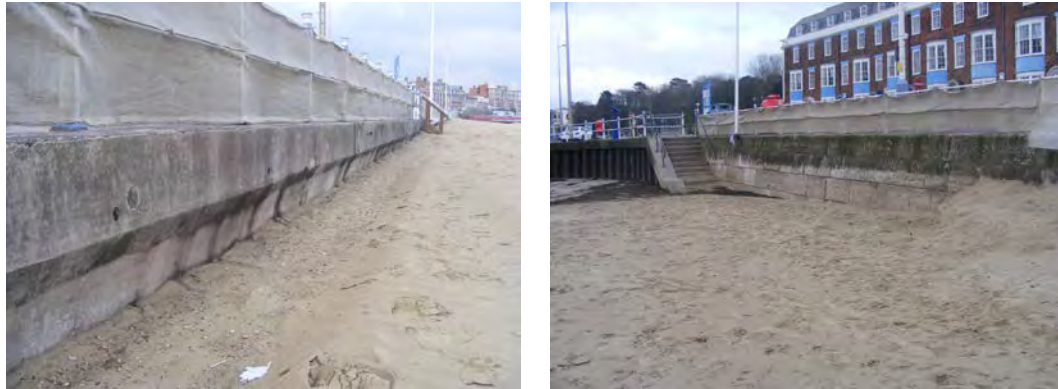
Figure 3-8 (left) photo of the concrete wall that runs for most of the length of the frontage south from Jubilee Clock to the Pavilion Peninsula; (right) photo of older masonry block wall not replaced with concrete in vicinity of Alexandra Gardens where it transitions to the steel sheet pile wall of the Pavilion Peninsula (23-11-2018; photos by A. Frampton).
