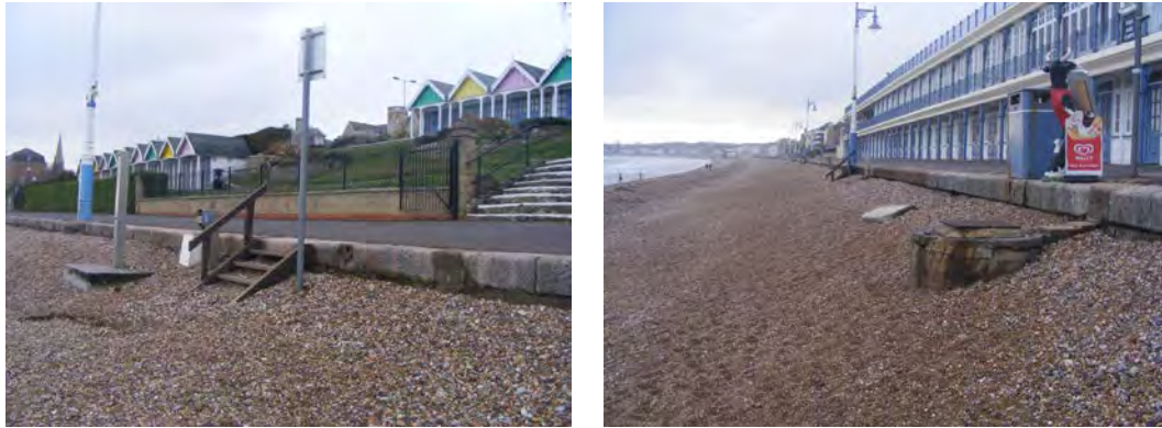
Figure 3-6 Photos of the promenade/seawall along the Greenhill Beach section of frontage, between Greenhill Groyne and Greenhill Gardens (23-11-2018; photos by A. Frampton).
