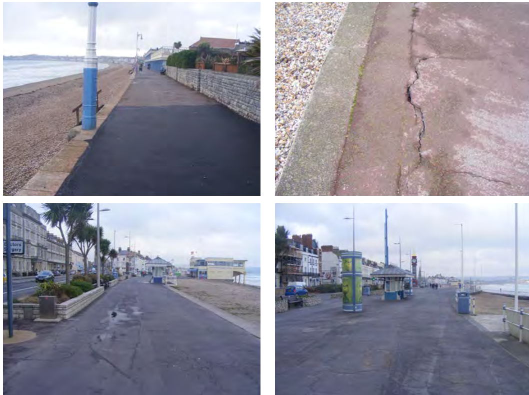
Figure 3-16 Photos showing uneven surface along parts of the promenade, and recent repairs (top left) (23-11-2018; photos by A. Frampton).
