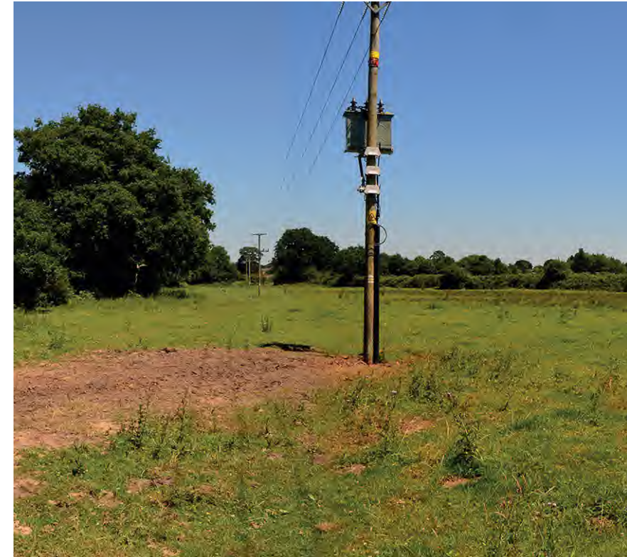
View looking north of overhead cable travelling southwards across the eastern parcel
