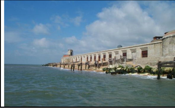
View looking approximately northwest of wooden groynes and rock revetment on south side of Hurst Castle, Hurst Spit.
