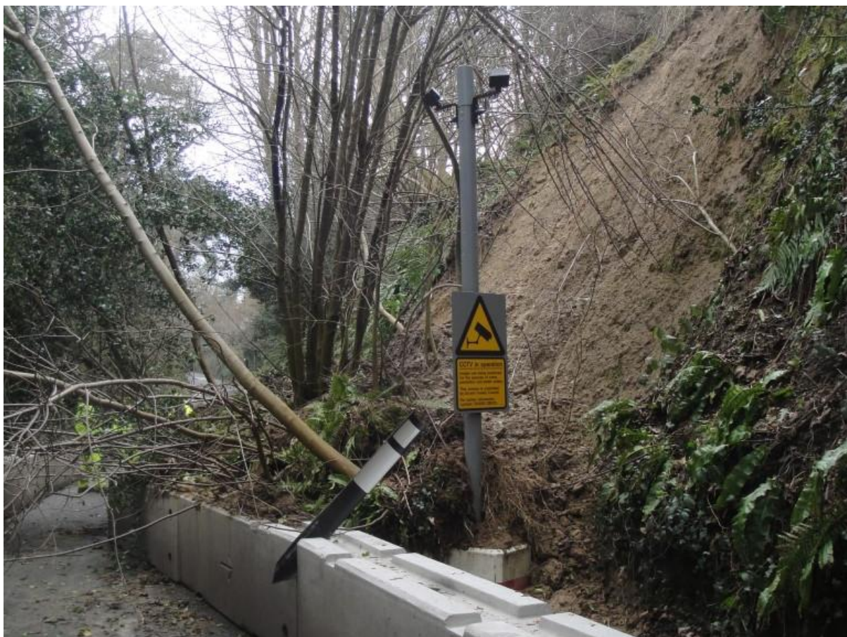
Figure 2: Landslip – viewing North
