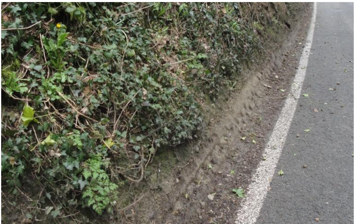
Figure 12: Tyre marks exposing soft material (approx. chainage 250, West)
