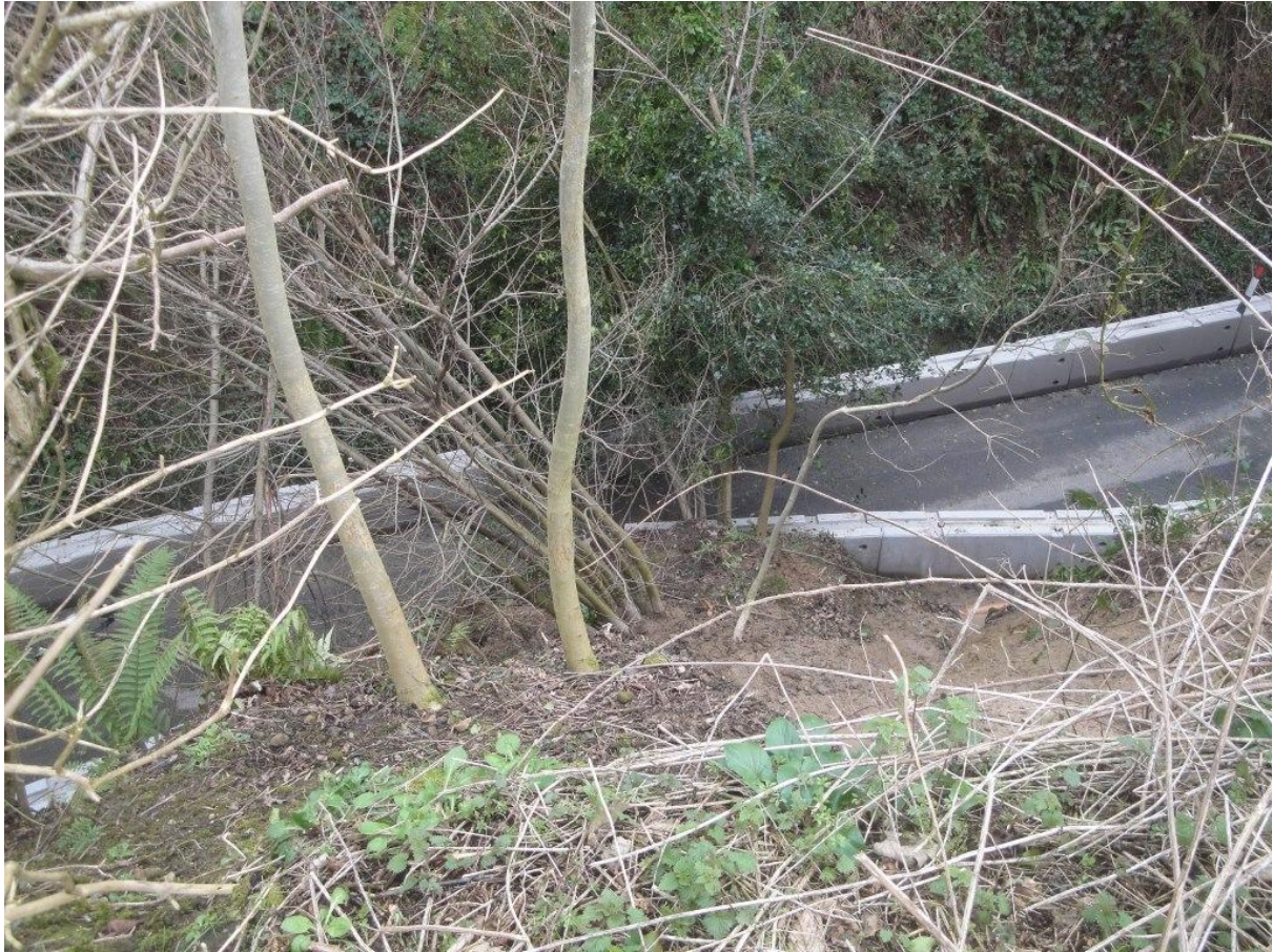
Figure 7: View from top of landslip
