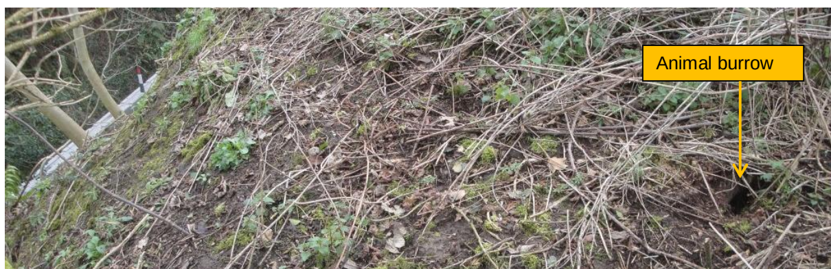
Figure 6: Ground above landslip
