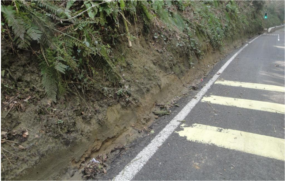
Figure 11: Wheel marks exposing fresh saturated sand (approx. chainage 250, East)
