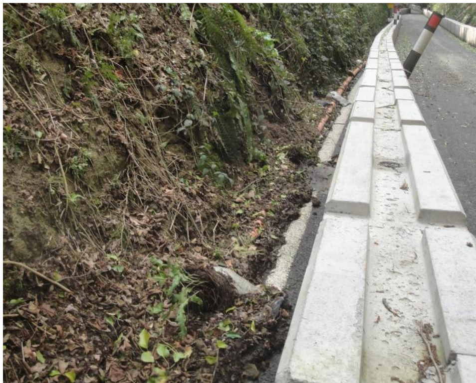
Figure 10: Material collecting at toe of slope (approx. chainage 180, East)
