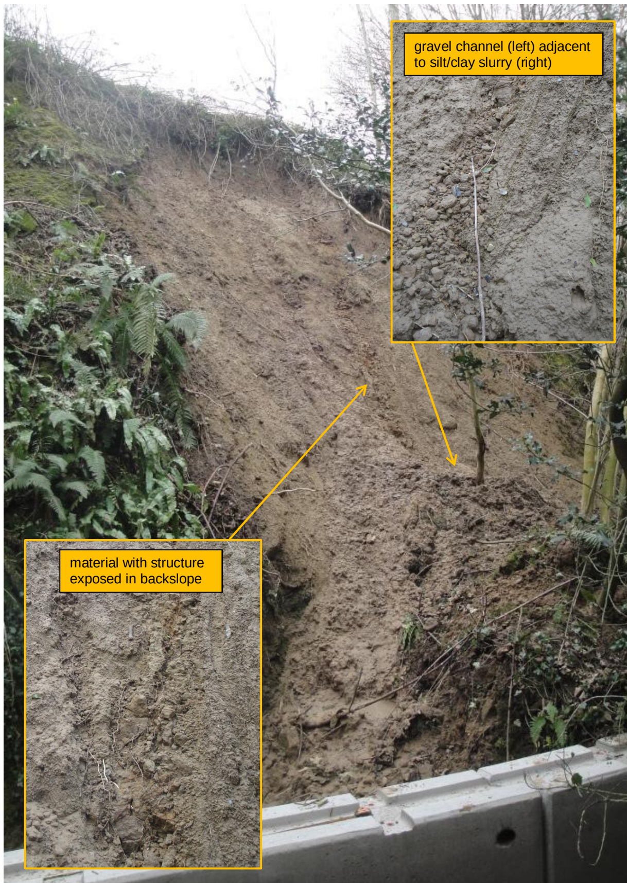
Figure 4: Backslope of landslide with features highlighted
