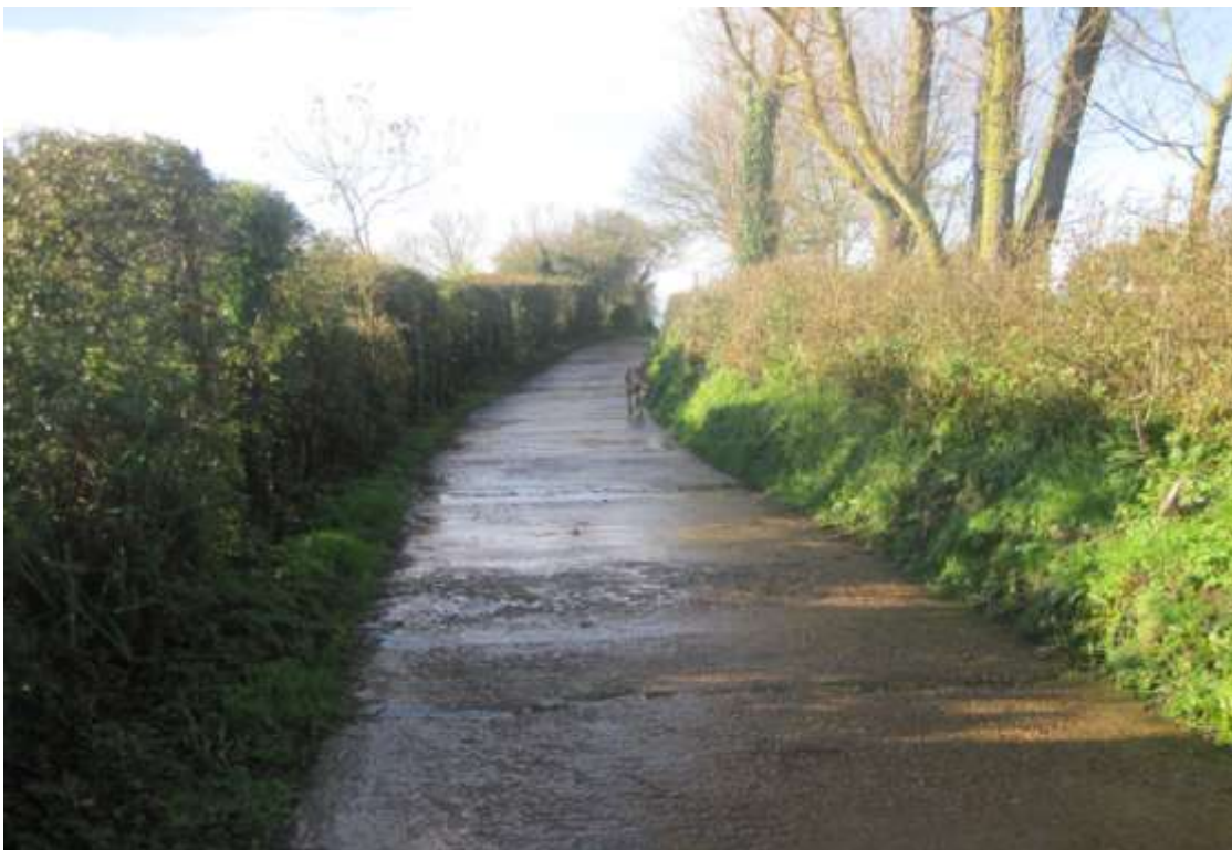
Section of Bridleway under dispute – concrete laid in 1943 still in place in 2015
