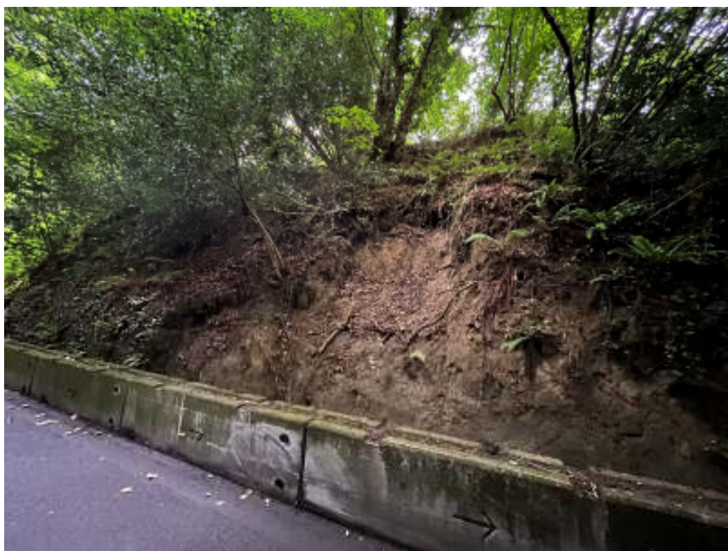
Figure 9. Evidence of recent slope movement, eastern bank
