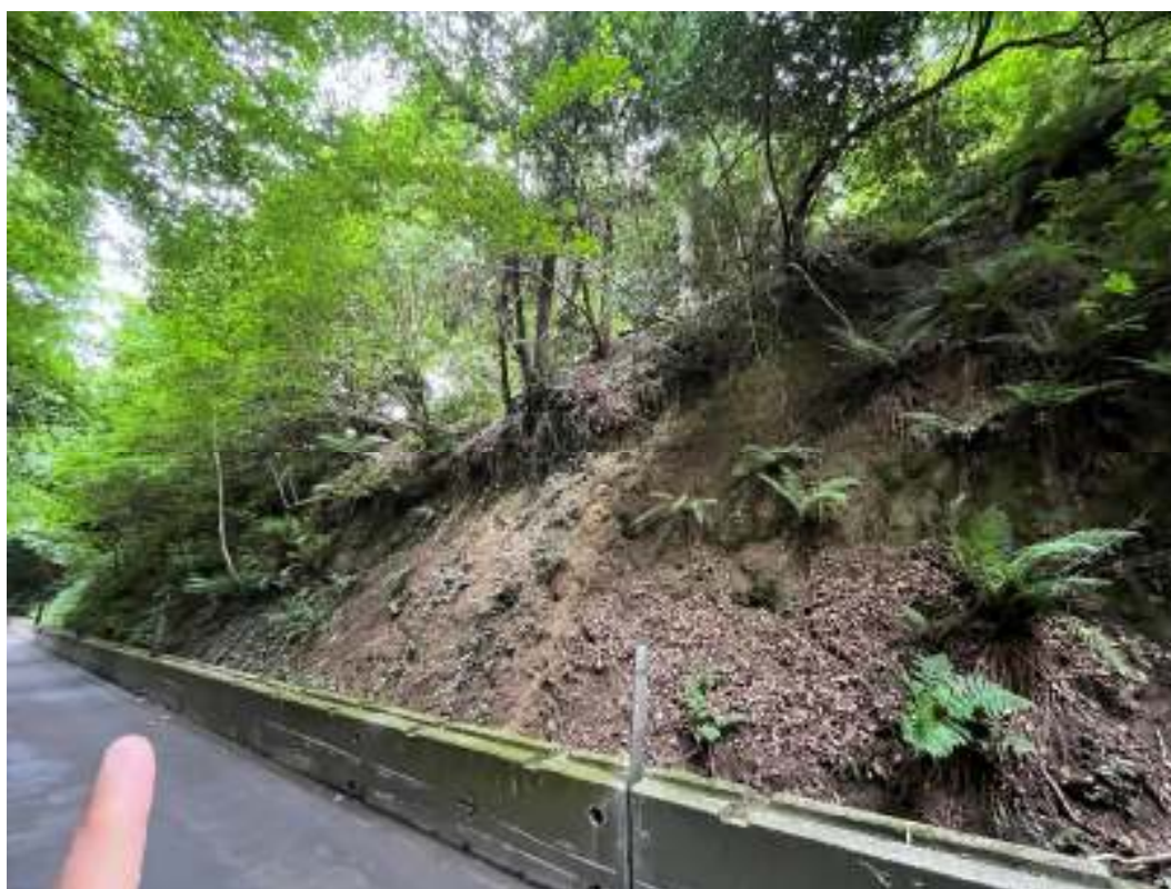
Figure 6 Possible indication of recent slope movement - limited vegetation and exposed tree roots.
