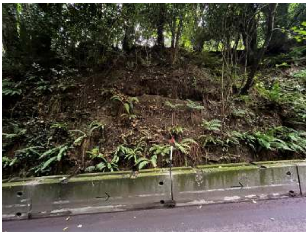
Figure 4 Evidence of back scar formation on the lower slopes, western bank.
