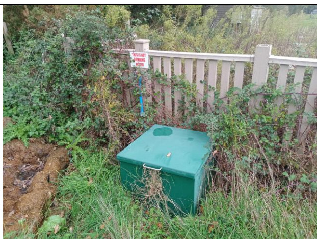
Photograph 11. Non-potable water storage in the north of the site.
