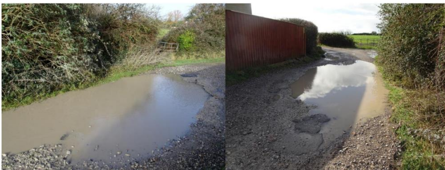
Corfehill Lane Flooding
