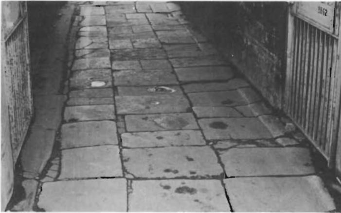
Wheel worn paving.
