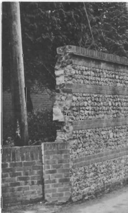
Severed walls should be properly finished off.
