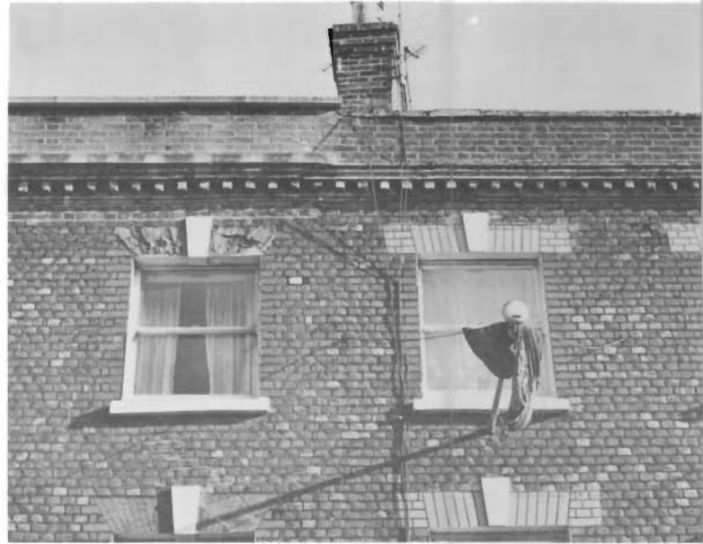
West Street window heads need careful repair.
