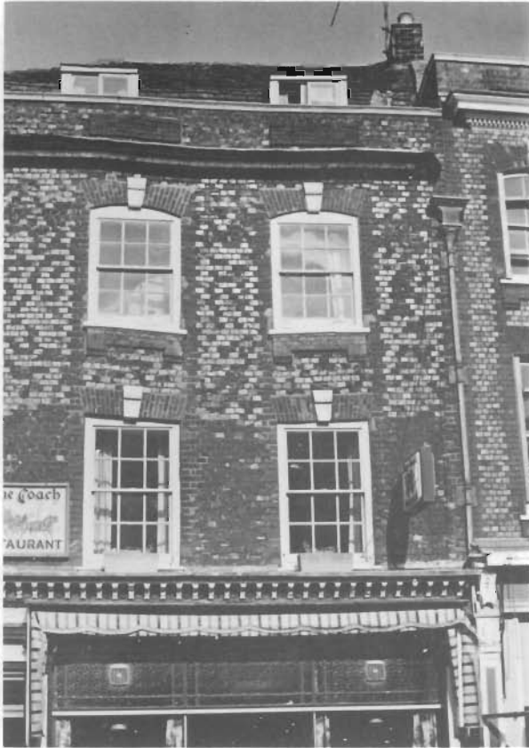
Sagging facade of No. 14 West Street.
