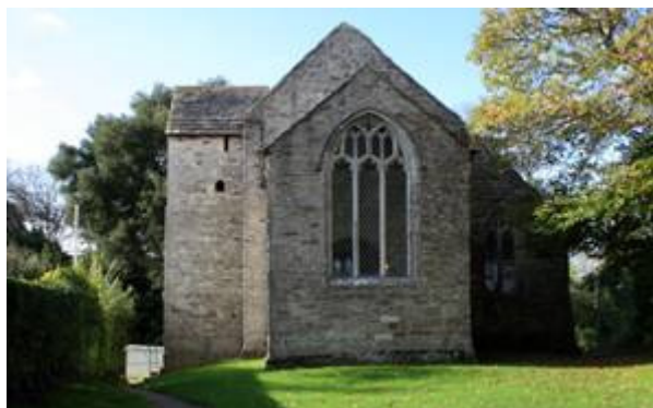
Figure 9: The east end of St Martin's Church showing the long and short stone work in the Chancel quoins.
