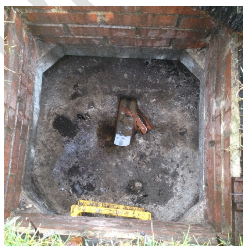
Figure 7 – Tankering location, taken on the 21/1/2015 when ground water was rapidly increasing and reached the trigger for preparedness.
