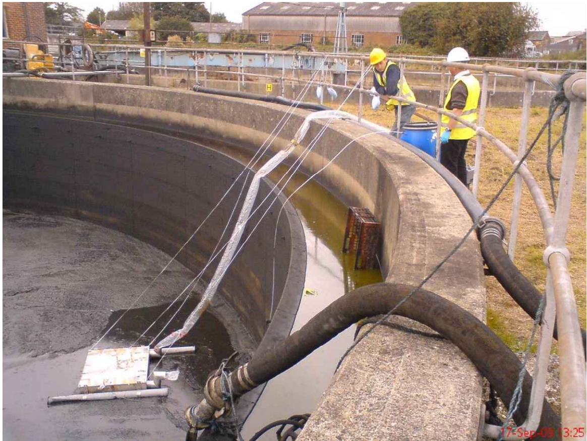
Fig 3, The Lindvall type hood collecting surface emissions from a sludge settlement tank.
