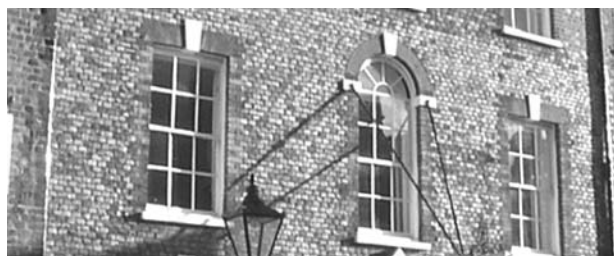
Fig 30. Example of vitrified header and rubbed and gauged brickwork on Barclays Bank
