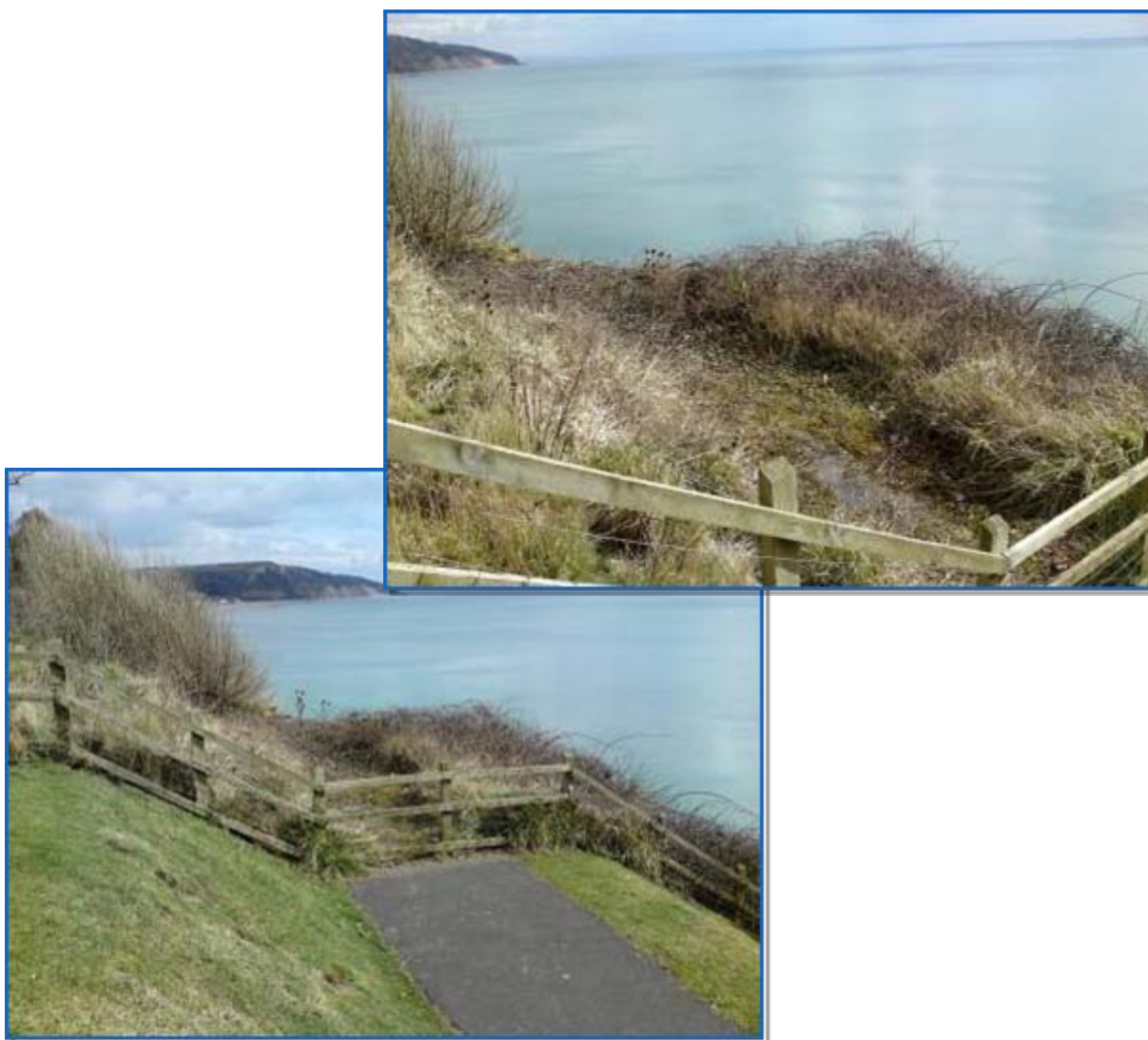
Eroded path at Seaton Hole leaving a path to nowhere.
