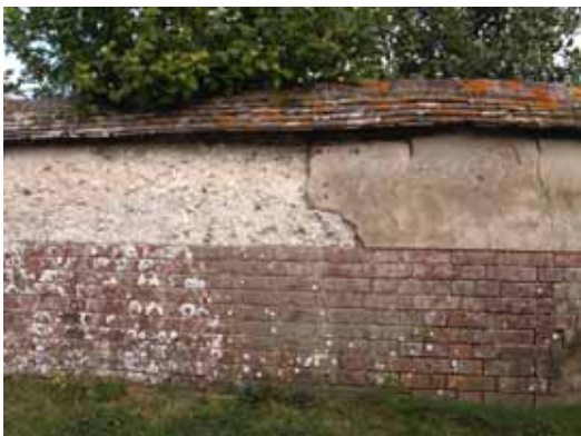
Chalk cob over a high brick plinth. Note failing cement render.
