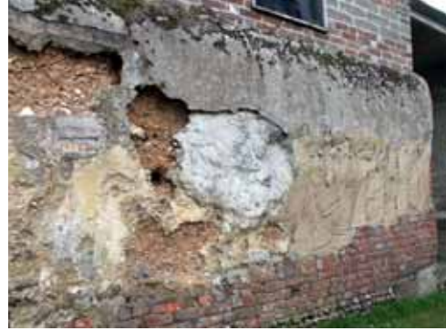
Erosion of cob made worse by crude attempts to patch up. Free-standing cob walls are particularly susceptible to neglect.
