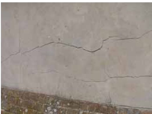
Initial signs indicating that things are not what they should be.
