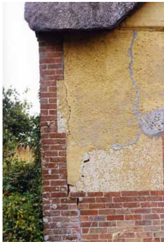
Here the brick and cob have parted company and the wall is bowing out.
