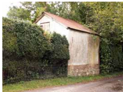
Cob implement shed on a plinth of brick over green sandstone and flint. Such buildings are becoming increasingly rare.
