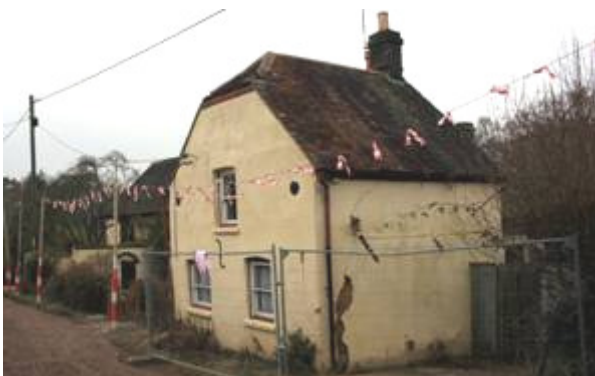
Figure 80: Number 2 Cobb's Road, Colehill. A recent crack in the wall has exposed the cob fabric.
