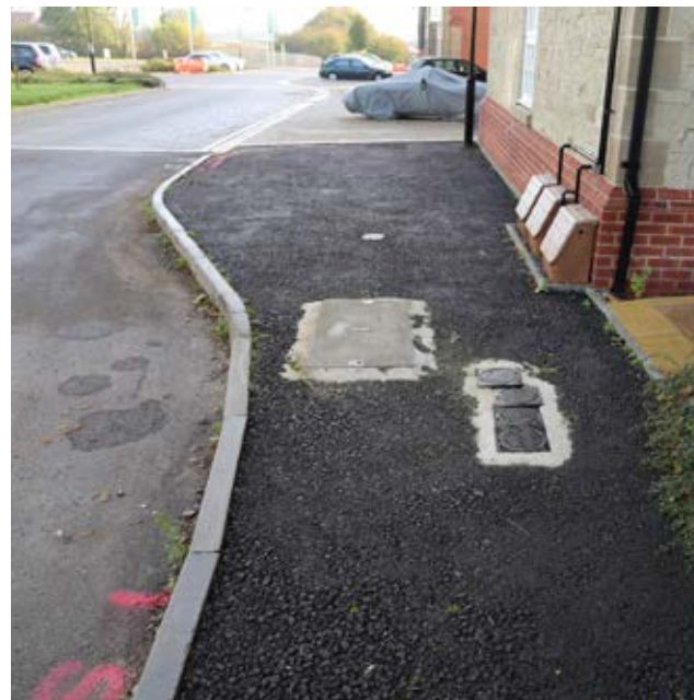
Poor quality road surface, Mampitts Lane
