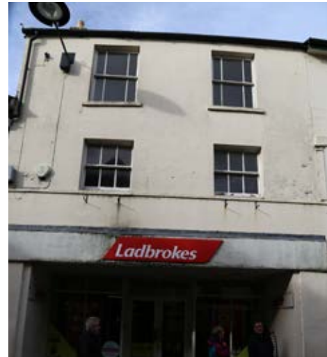
Poor quality shopfront High Street
