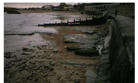
The depleted beach (above) will be replenished to protect the foreshore from attack by sea.
