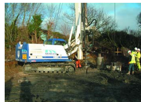
Over 1,000 piles will be inserted into the ground at Lyme Regis as part of the work.
