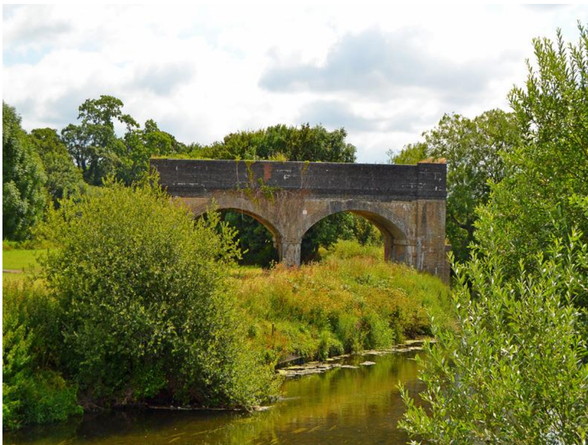
Figure 7.16: The remaining two brick flood arches of the bridge and embankment structure that formerly carried the railway over the River Stour
