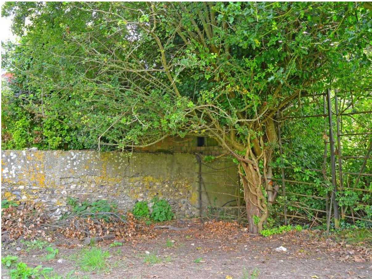
Figure 7.24: Brick and concrete pill box built partly on top of the wall at no.9 Parklands
