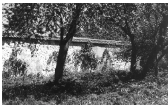
High chalk cob wall with Roman tile capping surrounding an old orchard in Long Crichel.
